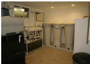
Bio-Matter Resequencing Converter, Greywater System and Enfinity Ozone and the first prototype Reverse Osmosis Disinfection and Filtration Recycling System
