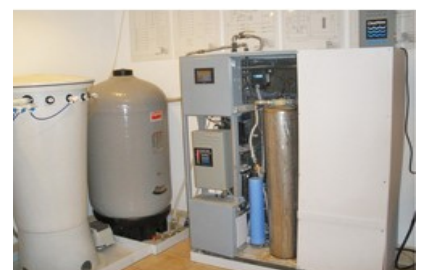
First prototype Ozone and Reverse Osmosis Disinfection and Filtration Recycling System
