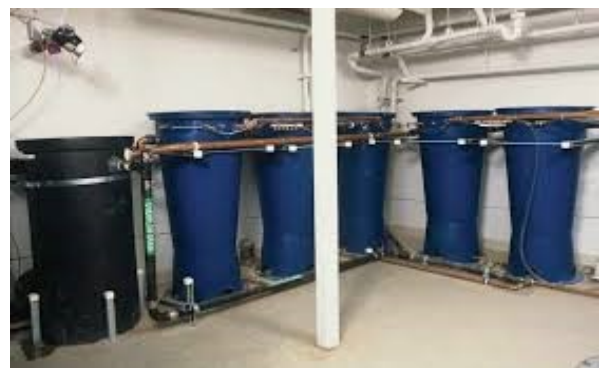
Two Greywater Treatment Systems installed at the Robert Redford Natural Resources Defense Council office building, Santa Monica, CA
