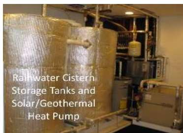
Rainwater Storage Tanks with Geothermal Ground Source Heat Pump
