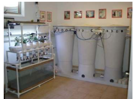
Aerobic Greywater Treatment System with Experimental Hydroponic and Aqua Culture System
