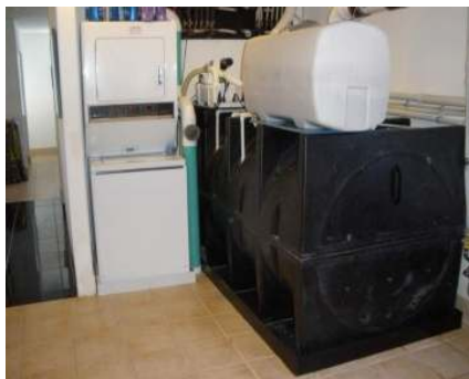
Bio-Matter Resequencing Converter—Composting Tank with Composting Tea Liquid Tank as a liquid fertilizer Resource
