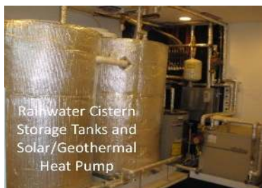
Rainwater Storage Tanks with Geothermal Ground Source Heat Pump
