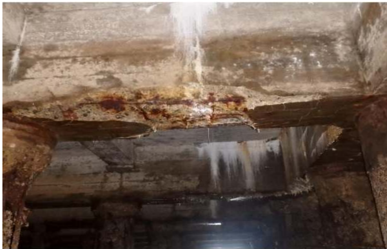
Figure 3-Corrosion and Spalling at Underside of Pier (Courtesy of Childs Report)
